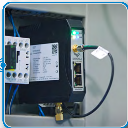
DATAEAGLE gateway inside the cabinet
